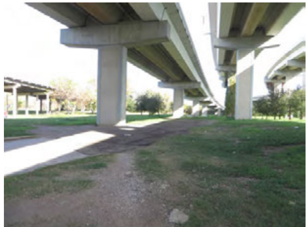
Figure 25. The APE under the US 59 flyovers, looking North. Note Elysian Street to the left
