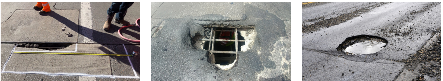
Figure 5: Existing Project Pavement and Bridge State of Repair
