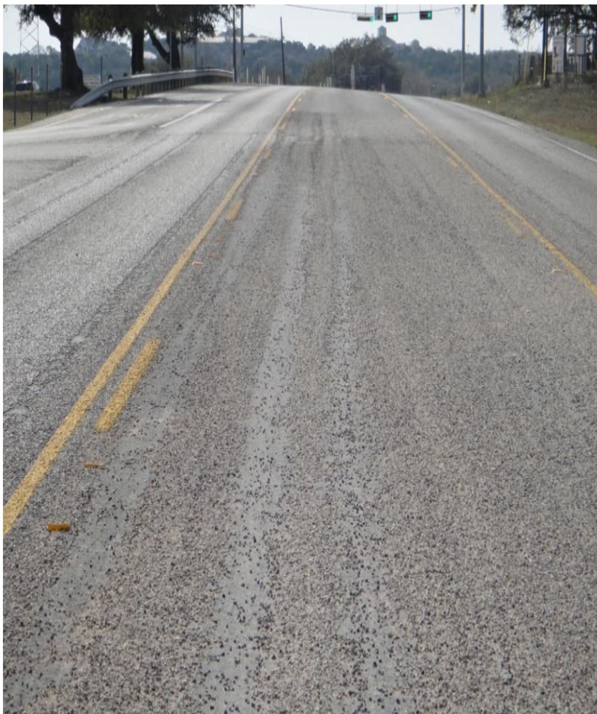
Figure 1-2. Seal coat pavement surface exhibiting aggregate loss.
