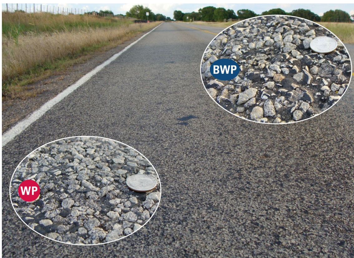
Figure 4-7. Lane with mild flushing.
