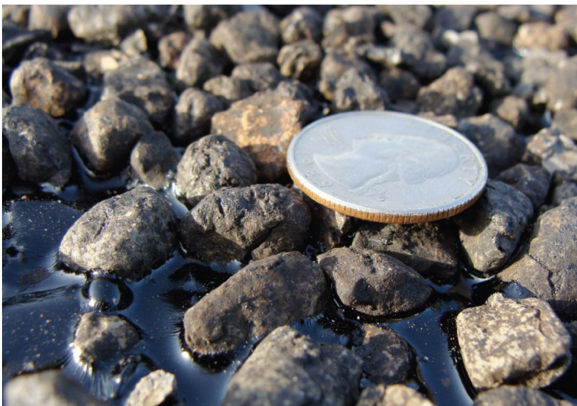
Figure 4-12. Wheel Path Aggregate Embedment Close-Up.
