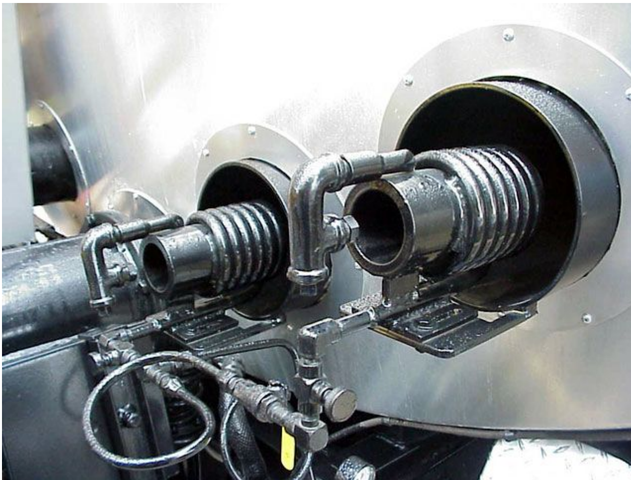
Figure 7-7. Burner Configuration at Rear of Tank.
