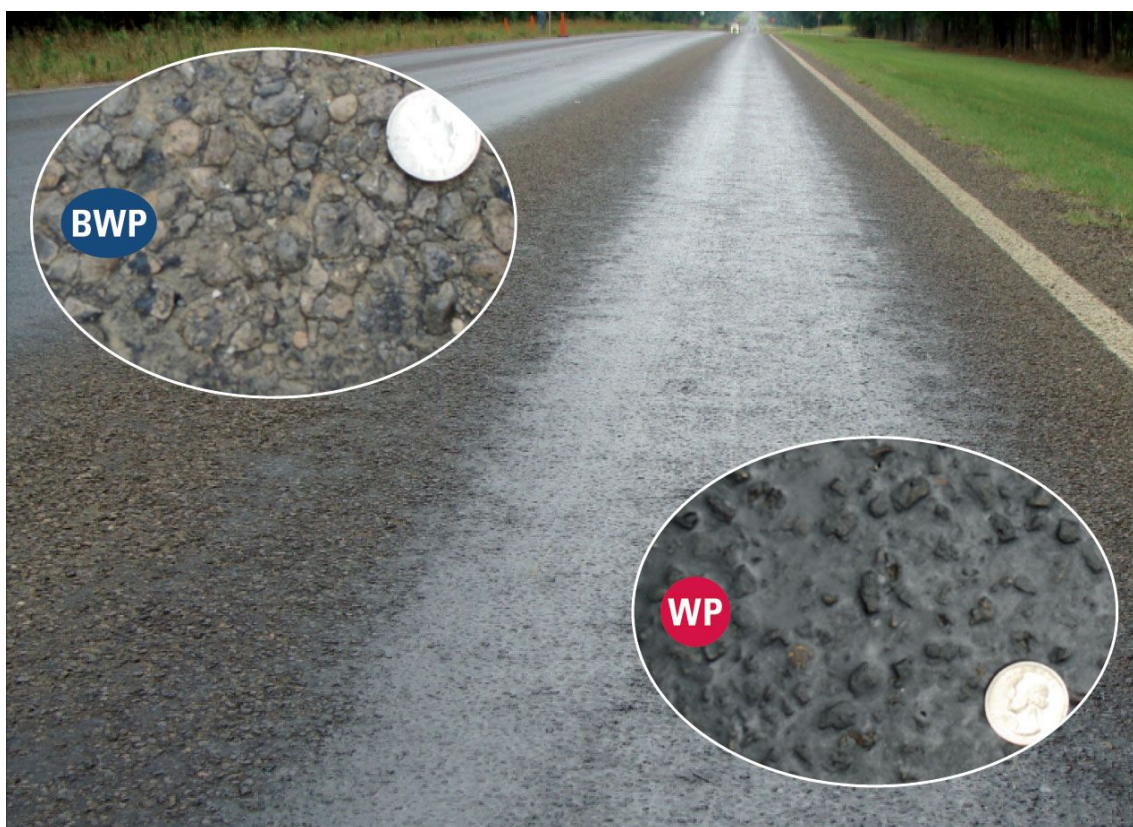
Figure 4-3. Lane with severe flushing. ♦
