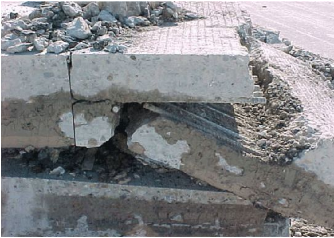
Figure 10-27. Construction joint failure.
