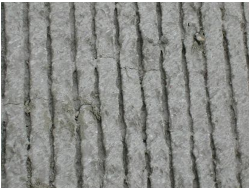
Figure 9-66. Plastic shrinkage cracks.
