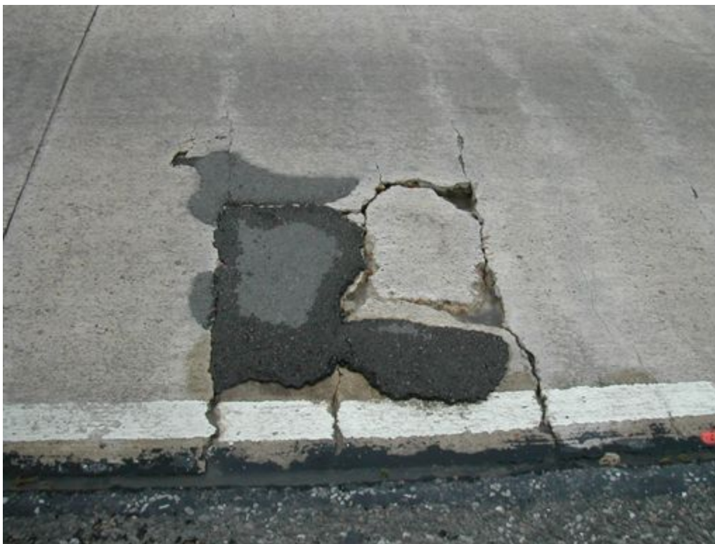
Figure 10-1. Typical punchout in CRCP.
