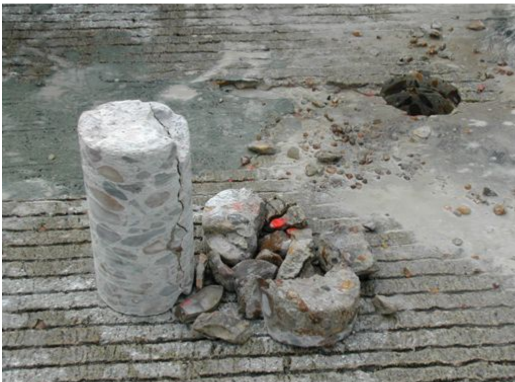
Figure 10-9. Coring adjacent to the spalled repaired area.
