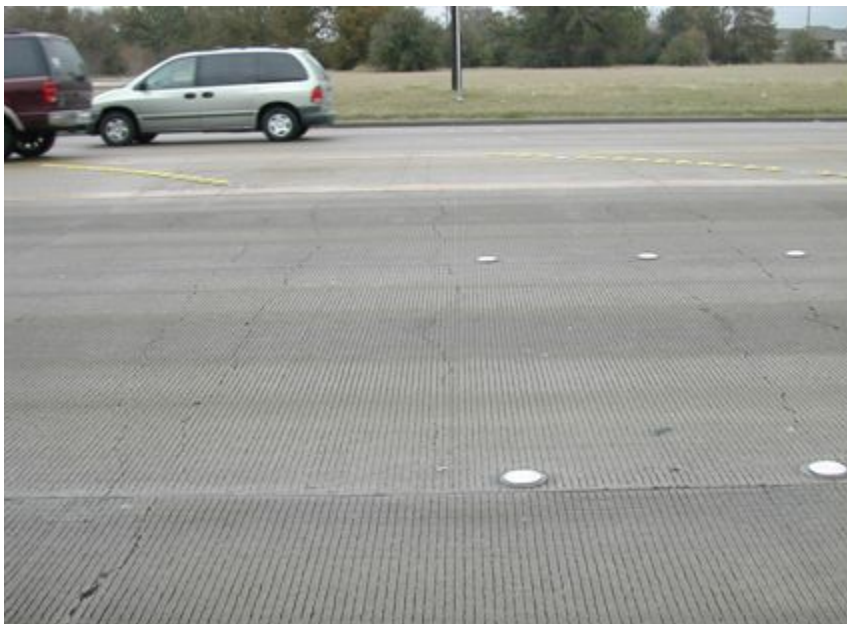
Figure 9-68. Random cracks in CRCP.
