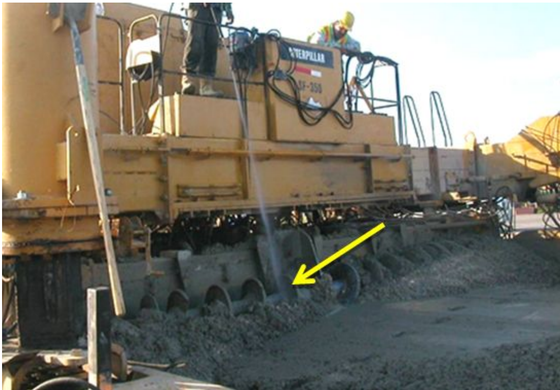
Figure 9-57. Unacceptable - Water being added.
