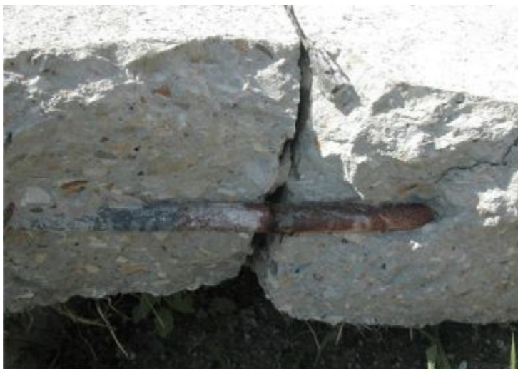
Figure 10-25. Rusted dowel bar.
