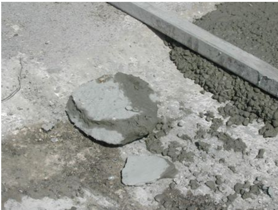
Figure 9-13. Large clumps of concrete.
