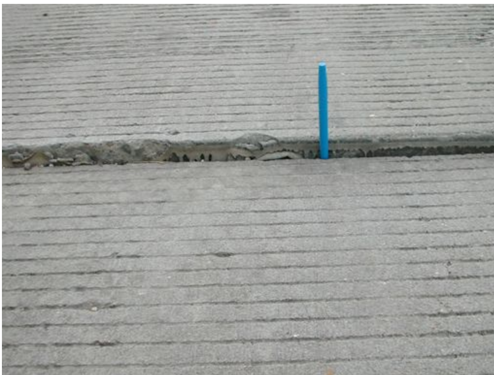
Figure 10-17. Severe faulting at the transverse joint.
