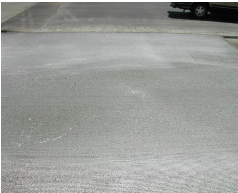
Figure 9-65. Unacceptable – non-uniform application of curing compounds.
