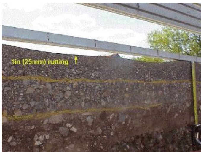
Figure 4-17. Trench sidewalls showing severe rutting.
