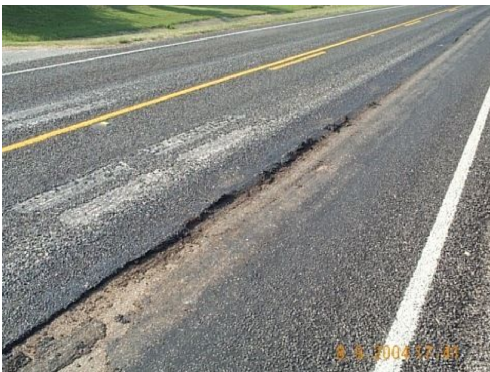
Figure 13-7. Peeling of fresh seal coats (2nd photo).
