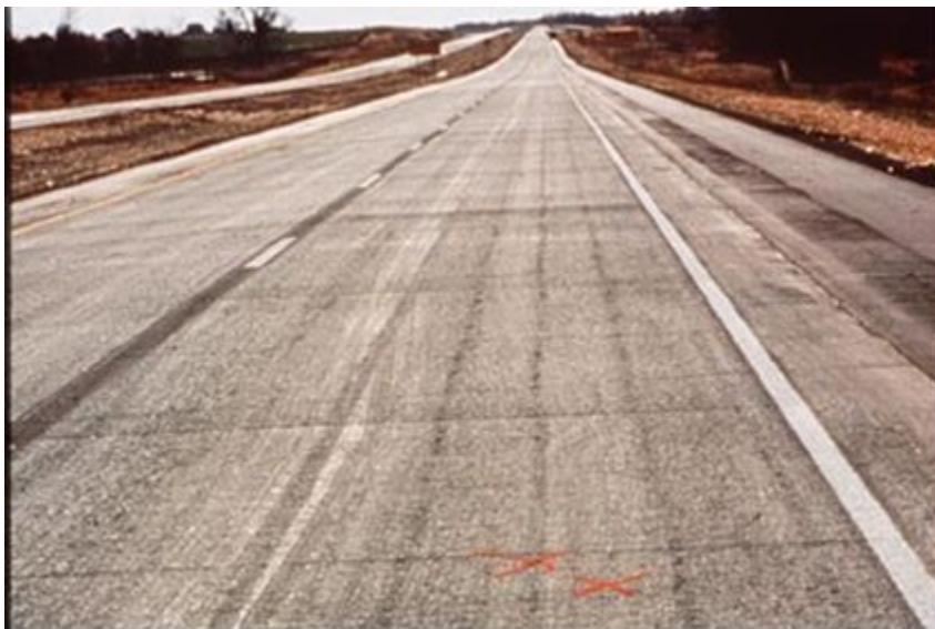
Figure 9-48. Unacceptable – vibrator streaks.
