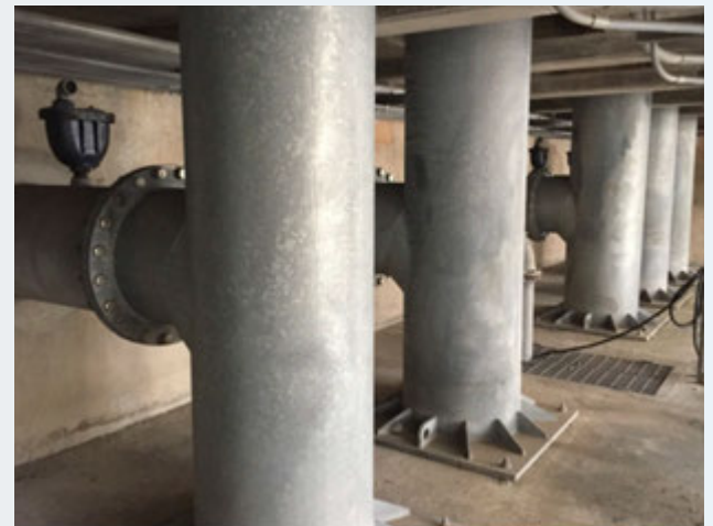
Pump Discharge Pipes.
