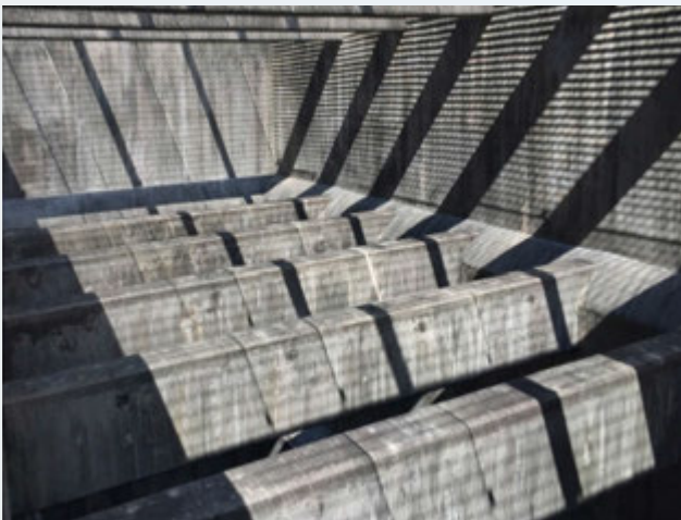
Upper Wet Well.
