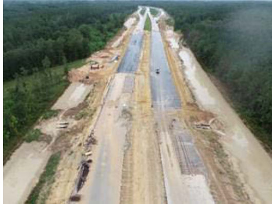
Figure A.1: Segment H1C After Tropical Storm Nicholas
