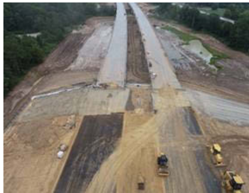
Figure A.2: Caney Creek Tributary After Tropical Storm Nicholas in Segment H1B
