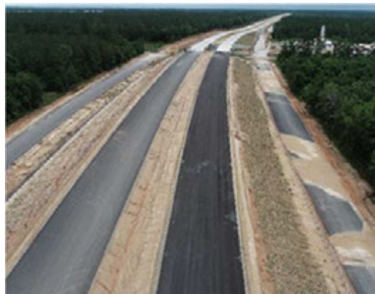
Figure A.3: Bond Breaker in Segment H1C
