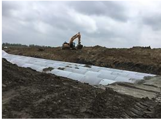
Figure A.5: View 96-in Pipe Installation at Luce Bayou in Segment H-1C
