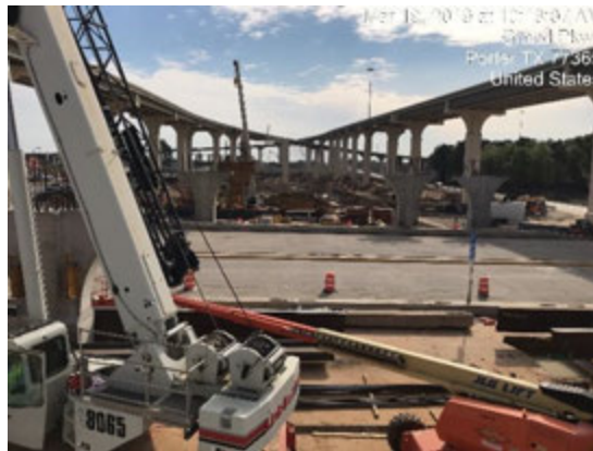
Figure A.1: View of Construction Operations at IH69 Looking East in Segment H-1A
