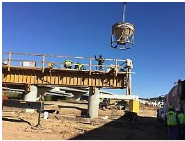
Figure A.2: Bridge 201, Bent 4, Concrete Pour at the Bent Cap in Segment 1
