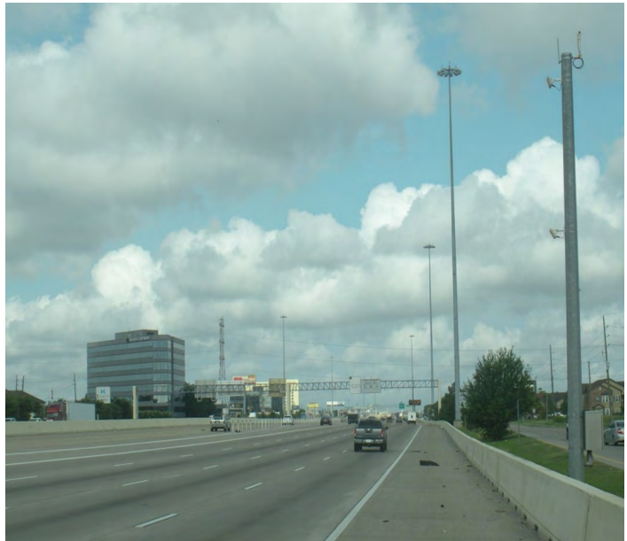
Sensors installed on IH 10 on pole.
