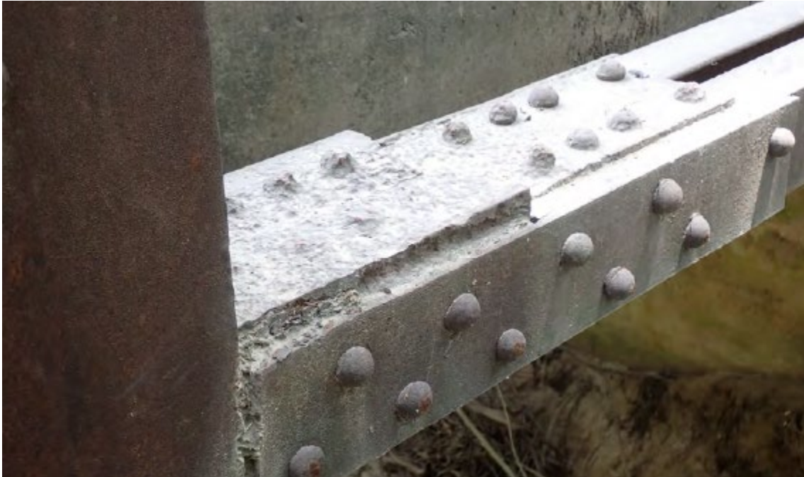
Photo 3: Corrosion at bottom chord with section loss
