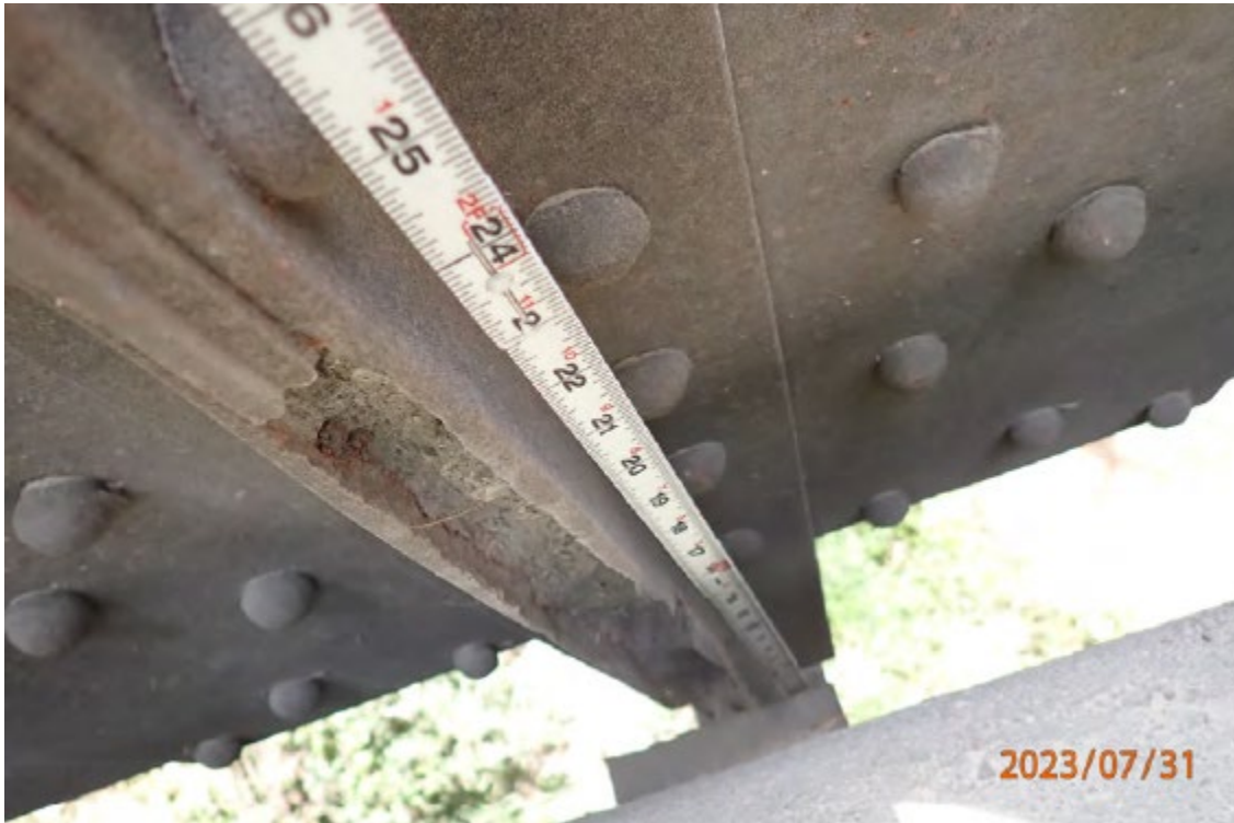
Photo 4: Pack rust on vertical members
