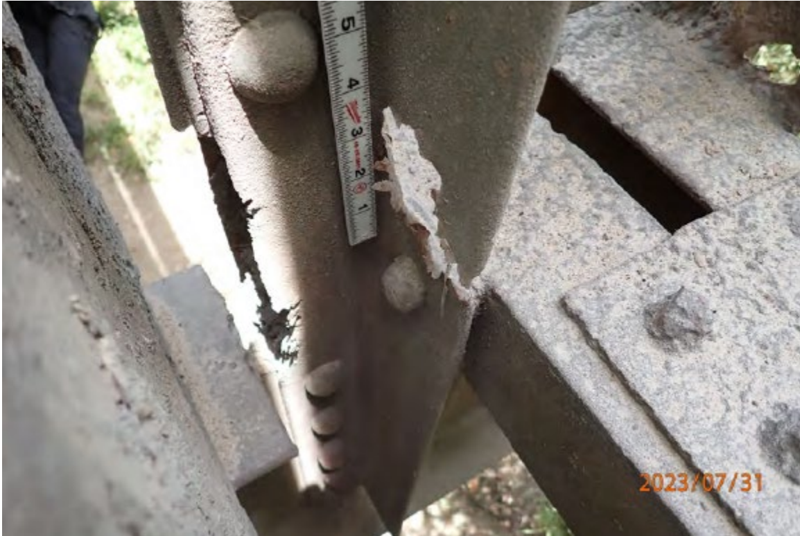
Photo 5: Section loss on vertical members
