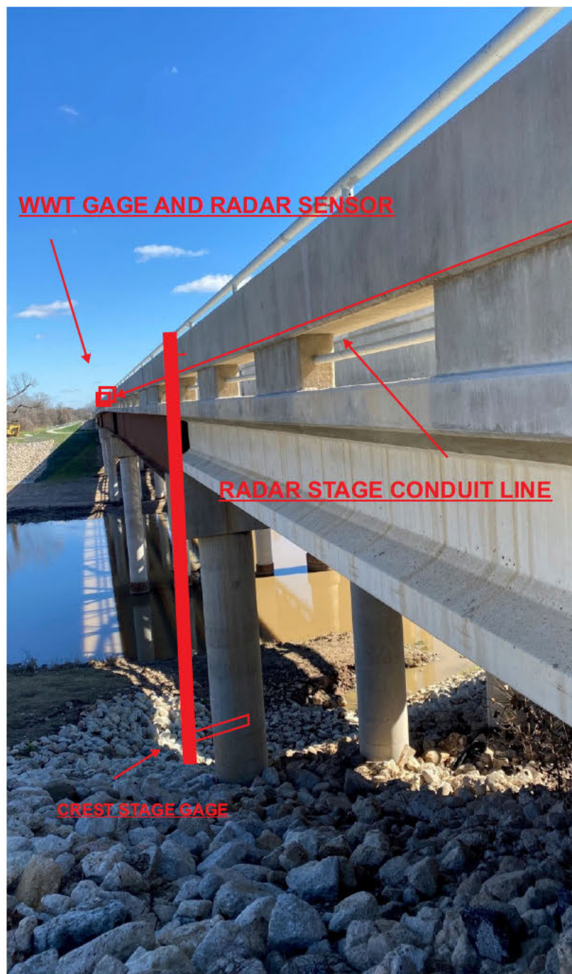
WWT, Radar Stage Sensor, CSG and conduit run at location.
