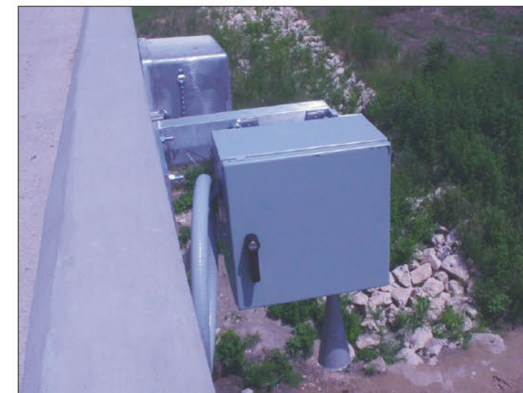
Typical installation of wire-weight gage and radar
