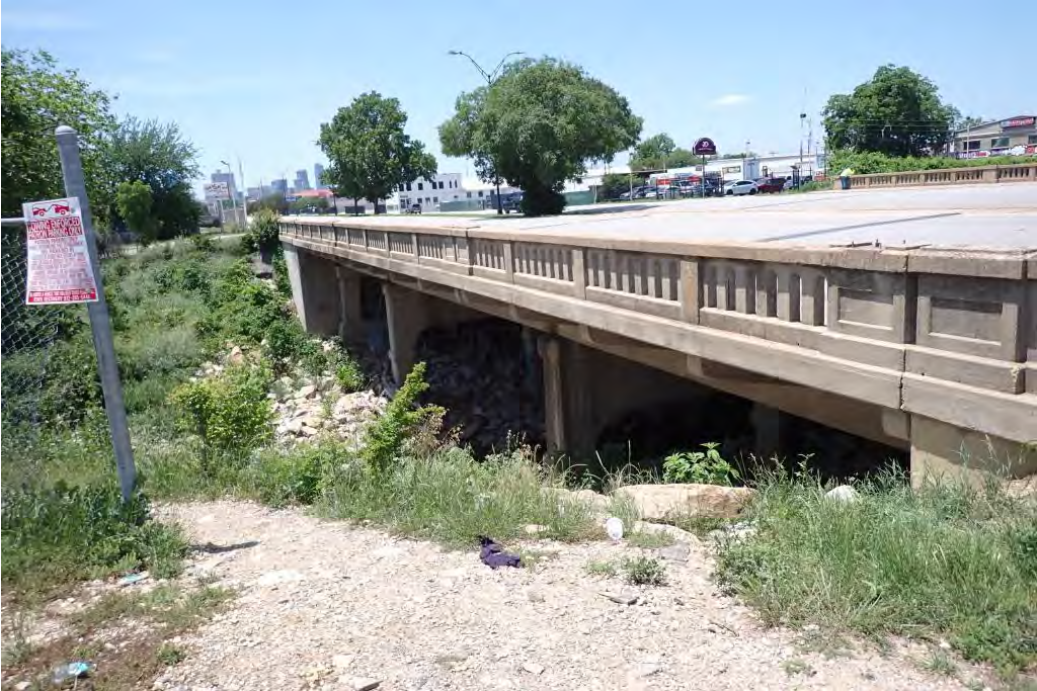
Figure 1. Side elevation of the SH 180 bridge over Sycamore Creek, looking northwest. TxDOT
