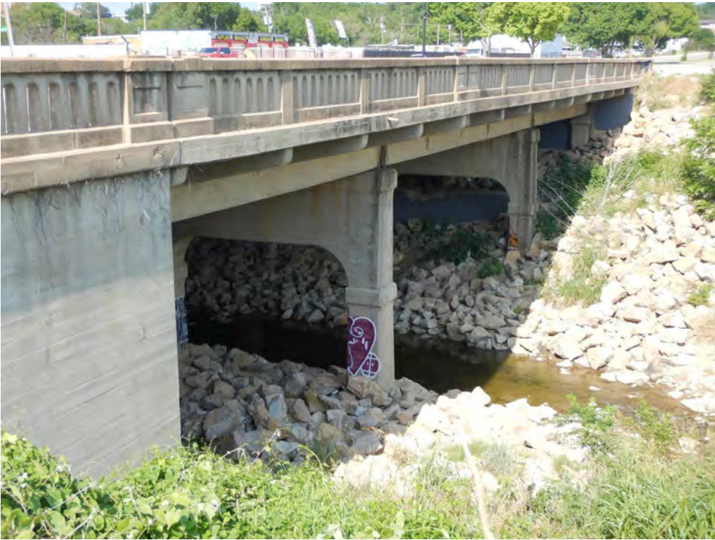
Figure 2. Side elevation of the SH 180 bridge over Sycamore Creek, looking southeast. TxDOT
