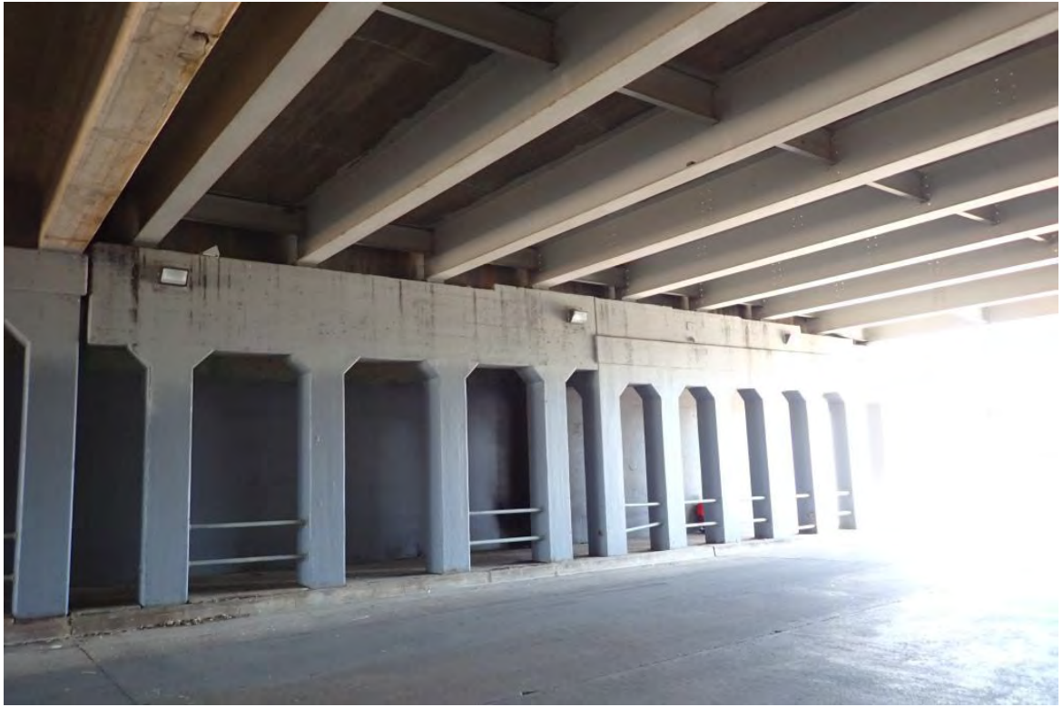
Figure 8. View of the underside of the State Highway 180 bridge over Harwood Street. TxDOT
