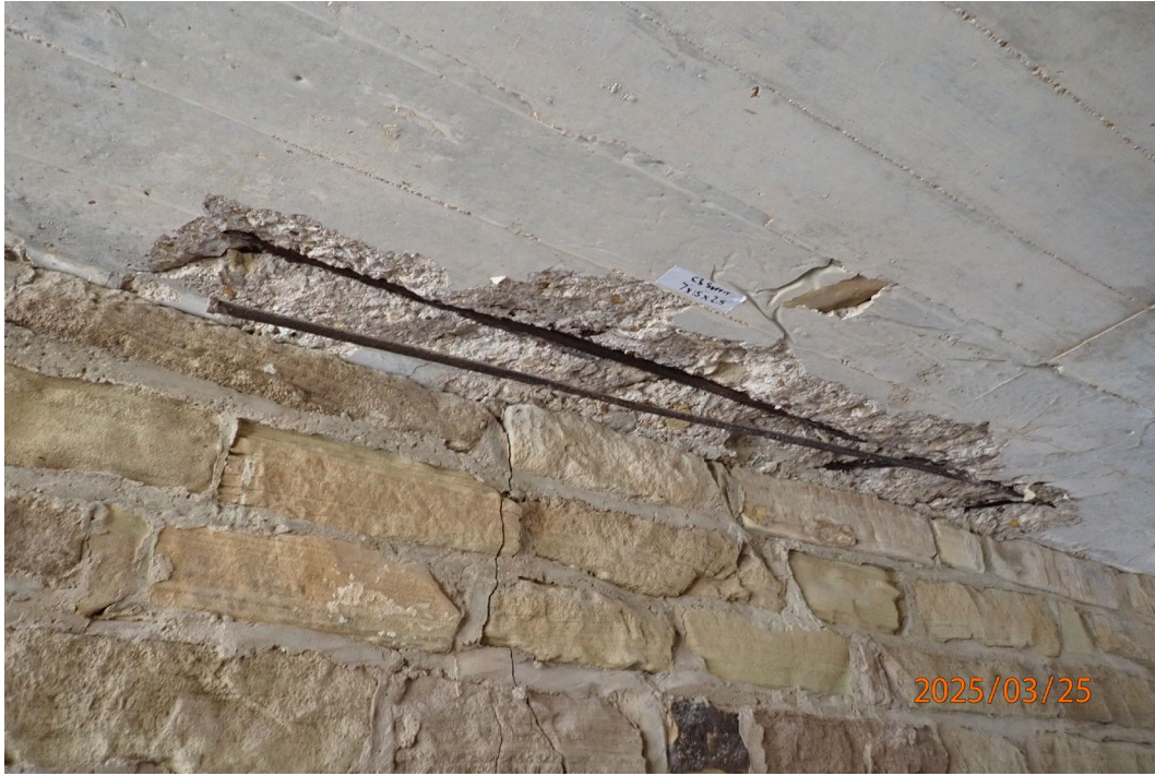
Figure 8. Photo of the underside of the slab with exposed rebar.
