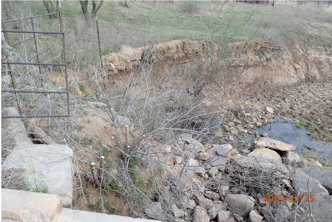
Figure 4. Northeast channel bank, showing erosion and stream migration.
