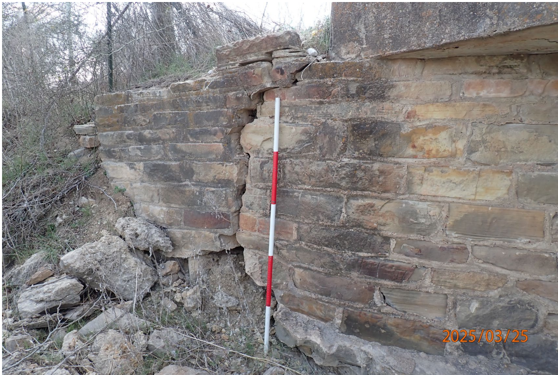
Figure 5. Southeast wingwall with vertical crack.
