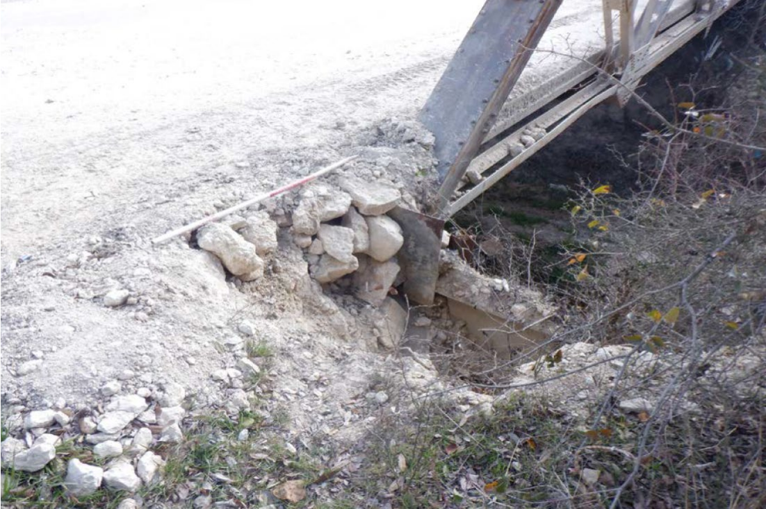
Figure 2. Erosion on northwest abutment.
