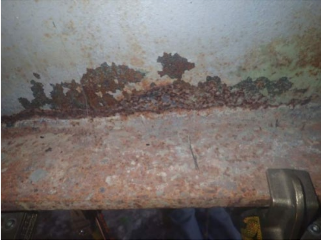
Figure 7. Photo showing paint loss and corrosion
