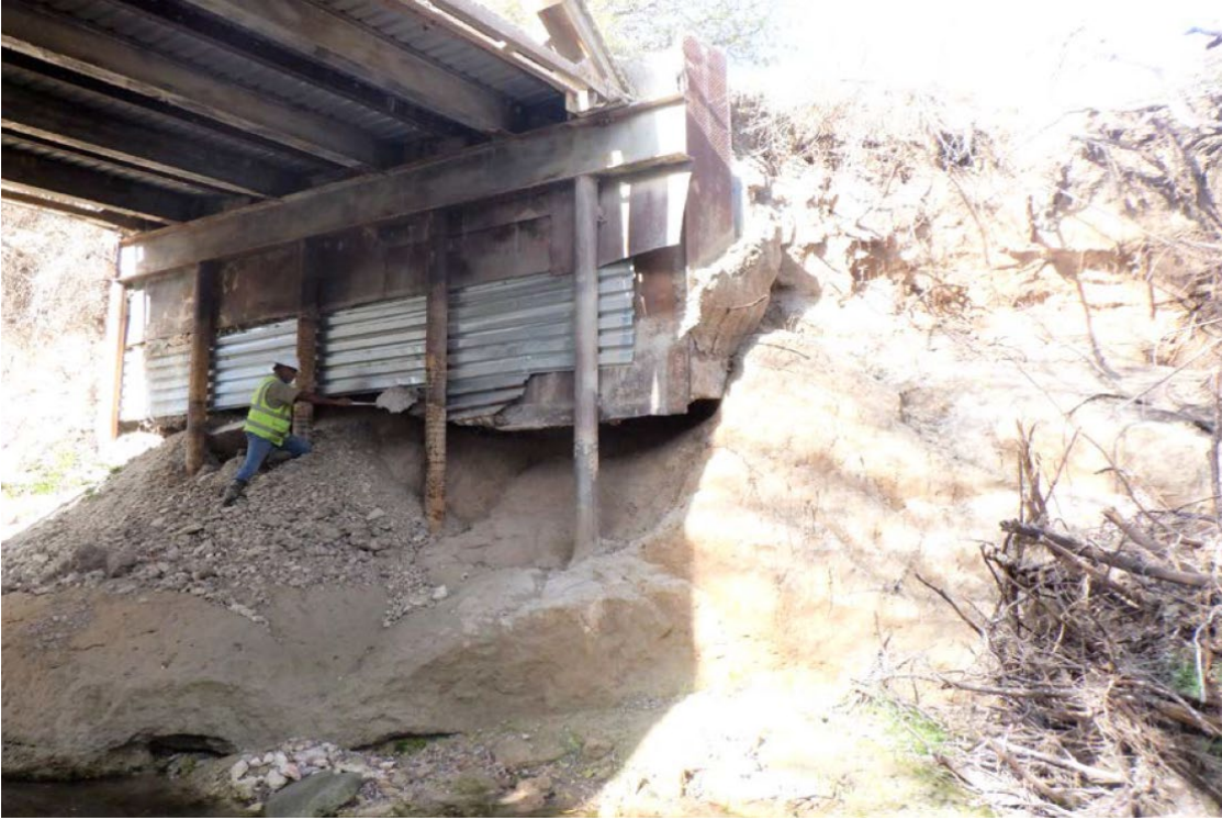
Figure 1. Erosion on abutment wall and pile exposure.
