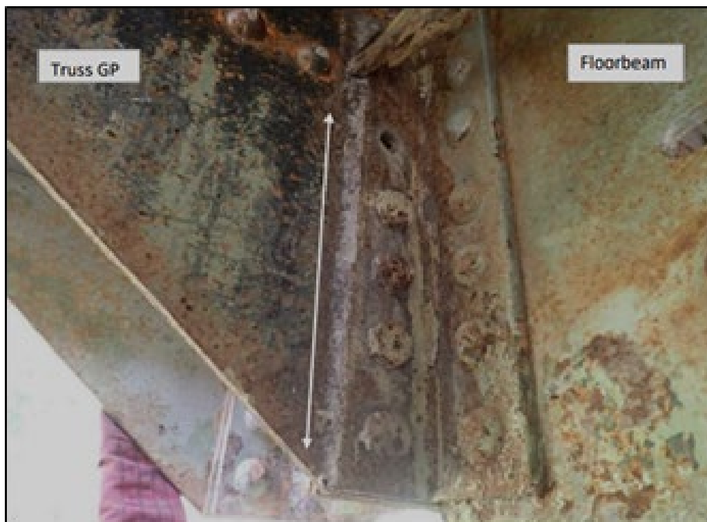
Figure 6. Photo showing missing bolts
