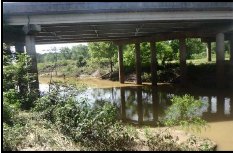
Appendix B – Photo 1: Chanel Spans of N Fork Taylor Bayou at IH-10
