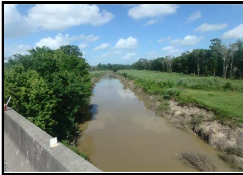
Appendix B – Photo 2: Downstream view of N Fork Taylor Bayou from bridge at IH-10
