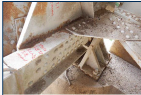
Severe corrosion on Gusset Plate around the Bearing
