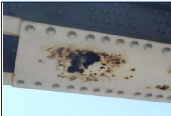
severe corrosion on lower chord batten plates
