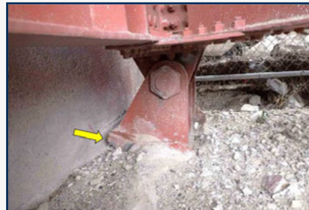
Excessive rotation (21.5°) of Truss bearing due to shifted rocker
