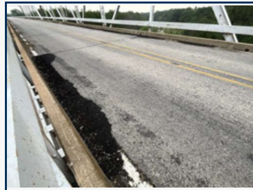
Poor Condition of Deck Riding Surface
