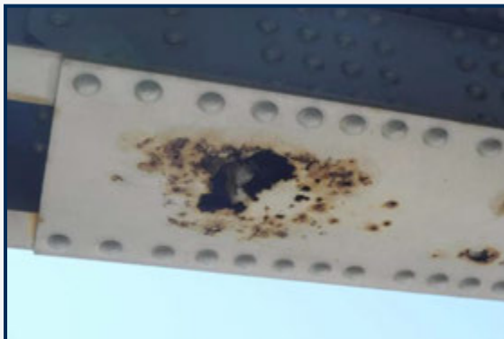
severe corrosion on lower chord batten plates
