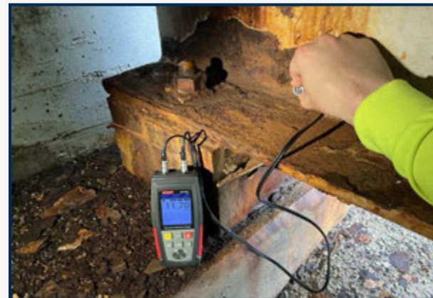
Corrosion with Section Loss in Floor Beam Web
