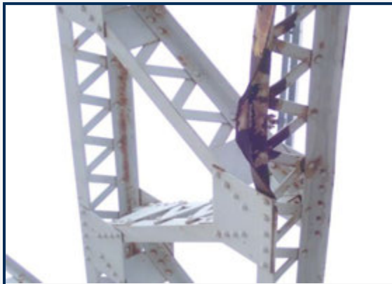
Impact Damage on Truss Bracing
