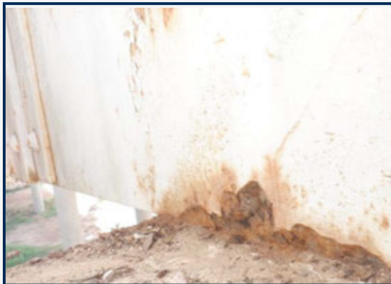
Severe corrosion on the Floor Beam around the Bearing
