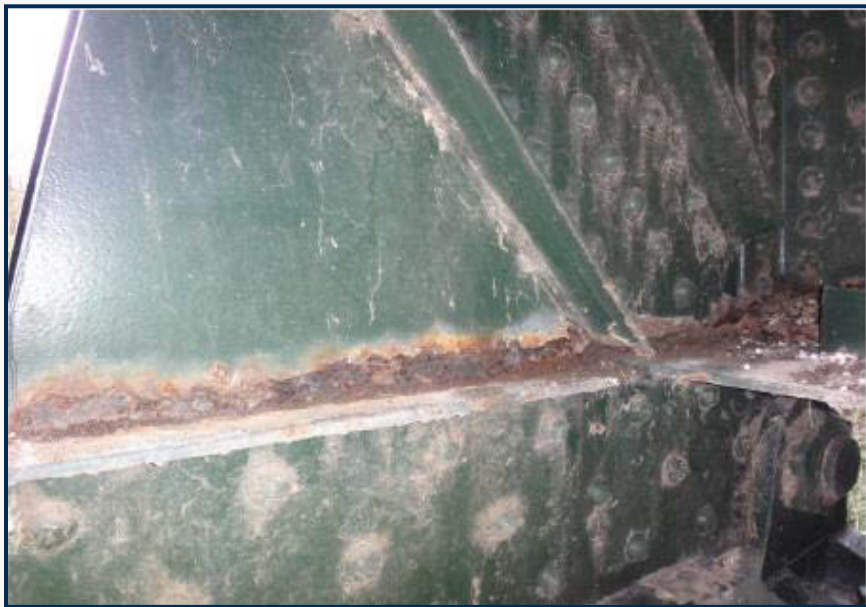
Up to 3/16" deep x 1" high x 30" long section loss to L0 inboard gusset plate along interface with a lower chord of the Truss (before blasting)
