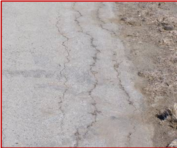
Figure 9. Cracked edges along pavement.
