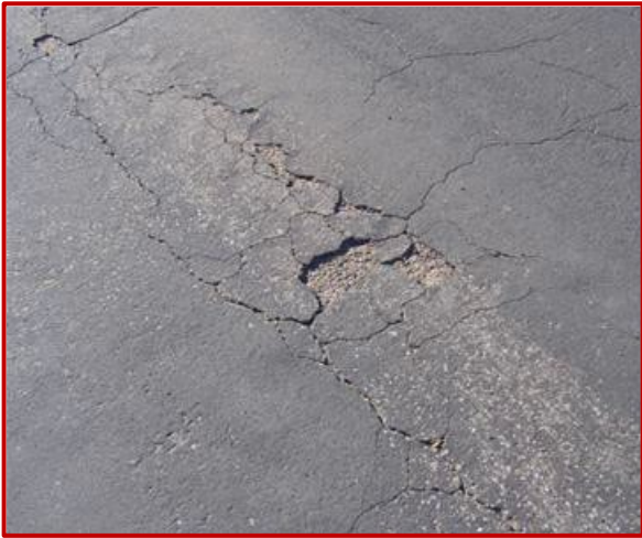
Figure 8. Pavement exhibiting spalling or shelling.
