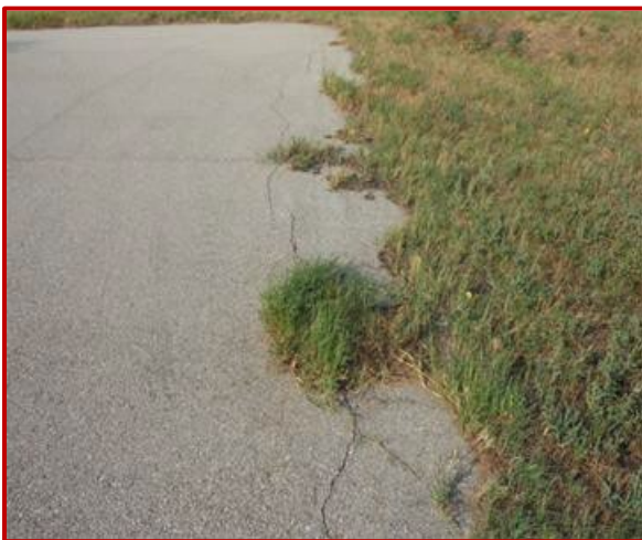
Figure 10. Grass growing through cracks in asphalt.
