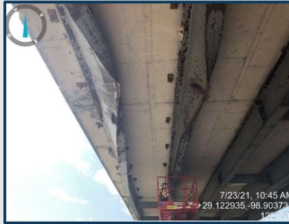
Overhead Impact damage
