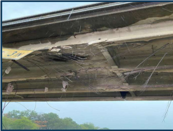
Overhead Impact damage
