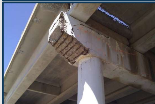
Spalling caused by deicing salt contamination
