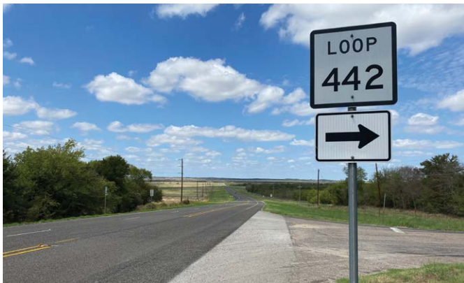
Texas Loop 442 in the Waco District still has its original pavement from 1929. Photos by Jake Smith
