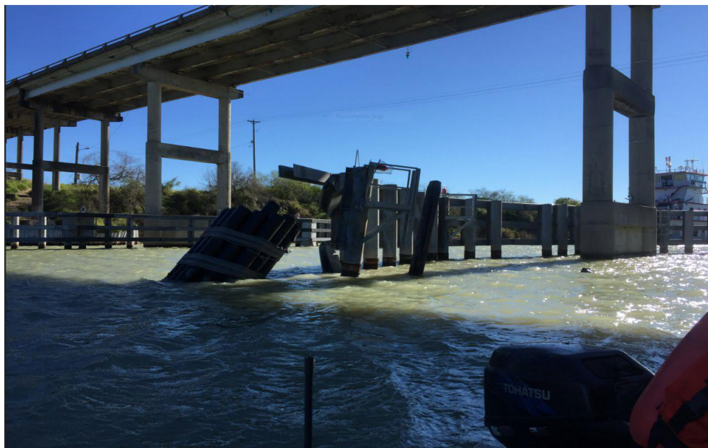
Figure 2-2 | Damage to Bridge Fender System, 2016 Crash
