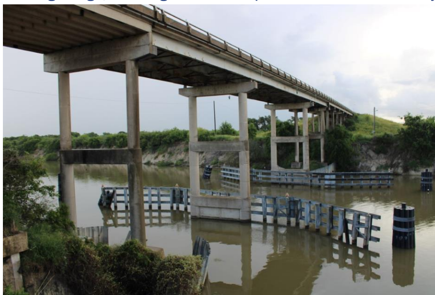
Figure 3-7 | Existing Bridge, Showing Corroded Superstructure and Fender System
