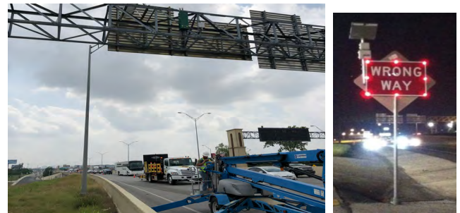
Video camera and detector with battery box and solar installed on OSB.
