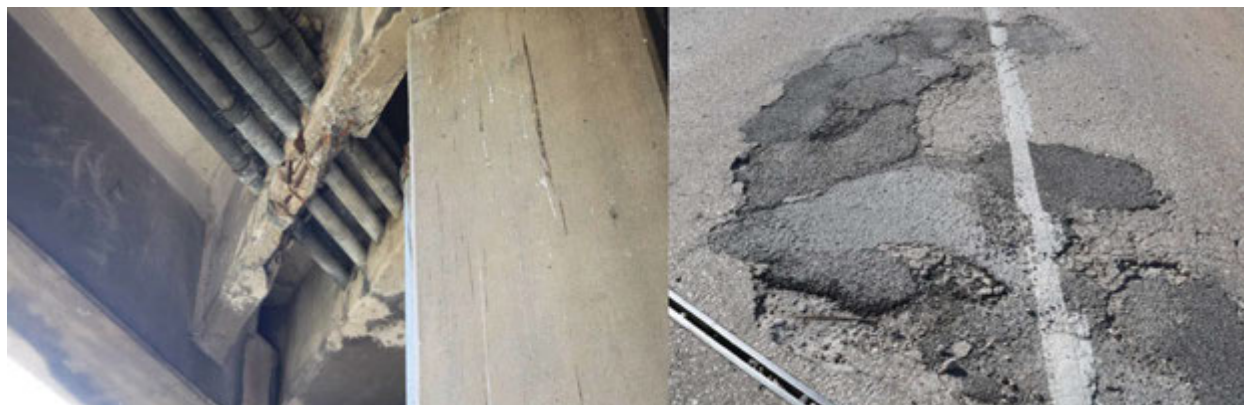
Figure 7 Corroded Reinforced Concrete and Deteriorated Bridge Decking
